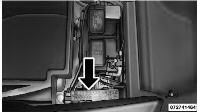
Rear Power Distribution Center
